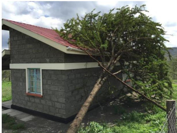
Figure 6: Collapsed tree on top of a RAPhouse
